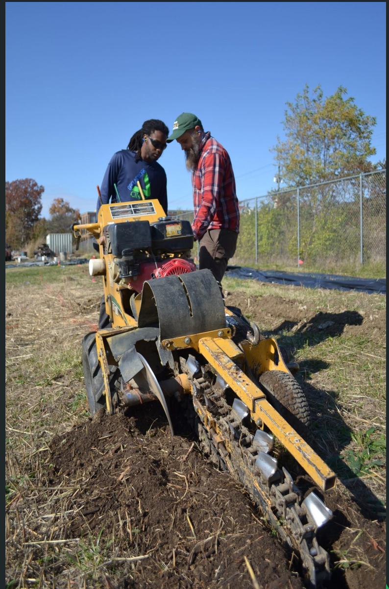
Anthony learns how to use a trencher in the building of an urban orchard
